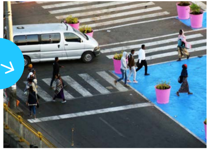
New crossings and pedestrian islands in the Sebategna intersection. © Glocal Designing Cities
